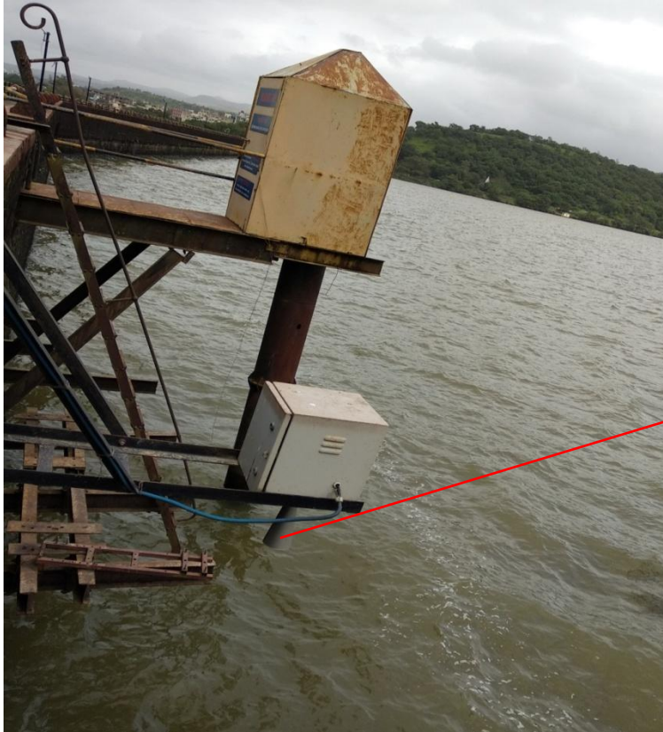
Radar Installed at Khadakwasla Dam
