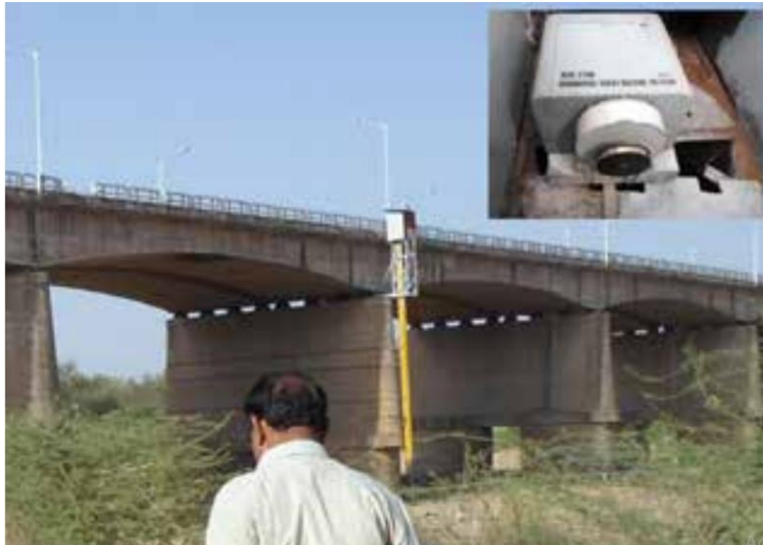
A shaft encoder installed on the side of a bridge in Gujarat
